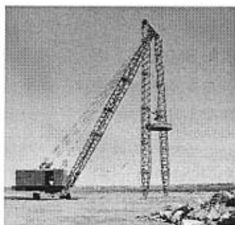
图 1.2-2 强夯机械及施工过程 Fig1.2-2 Dynamic compaction machinery and the construction process
